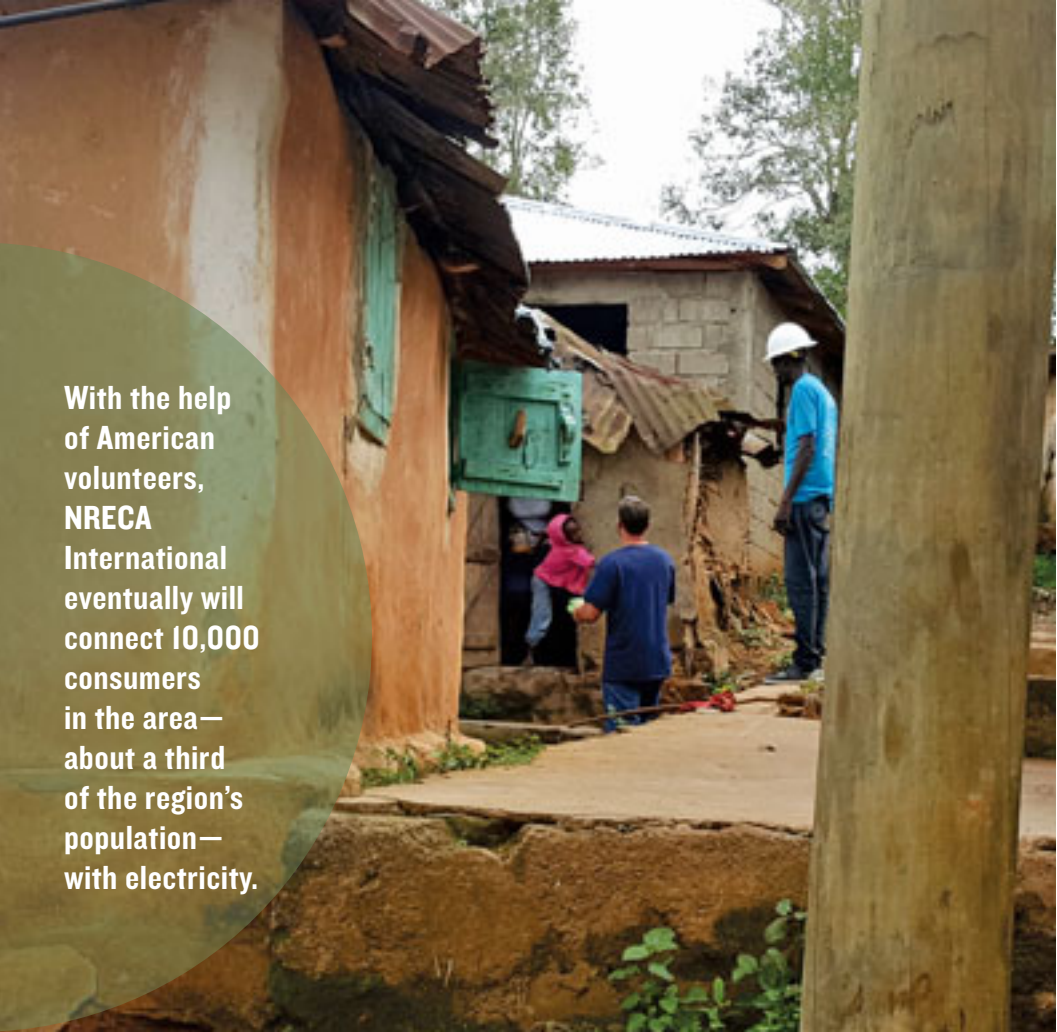
Mike Grisham hands treats to a girl who came out to watch his crew bring electricity to her home.
