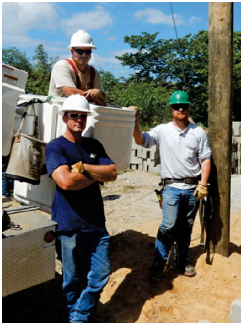
Opposite: Haitian and Texas linemen work together to bring electricity to Caracol. Above: HILCO EC's Mike Grisham, blue shirt, and Clayton Thompson, in the bucket, teamed with Brannon Nichols from Homer Electric Association in Alaska to build lines in Haiti.
